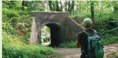
The bridge for the track along Benthall Edge from Bower Yard, which was cut off when the railway was built.
